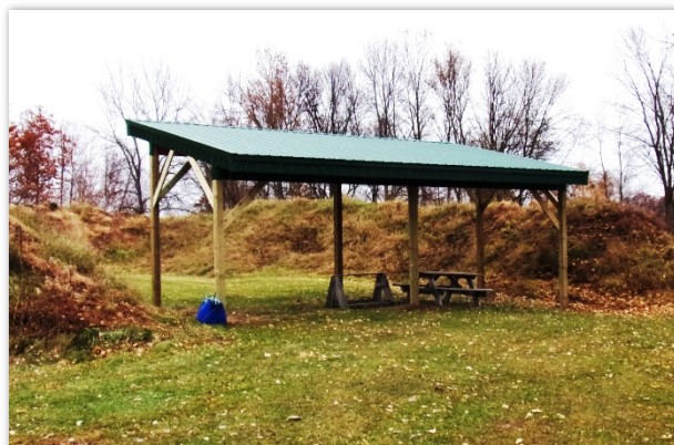
Figure 1: Pistol Range Shelter is up ...looking good! Thank you to Grandt Builders for donating the labor to get this structure up.
